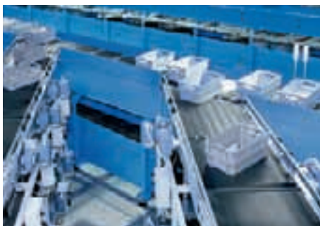
Letters correctly en route: Interroll cross-belt sorter with the Swiss Post Office in Zurich
