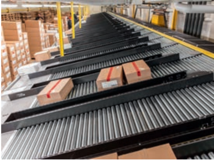
Just 52 hours: a success story of a sorter retrofit in 52 hours by Siemens and Interroll, during ongoing operation at the TKC Deep Freeze Logistics Center in Birrfeld, Switzerland.
